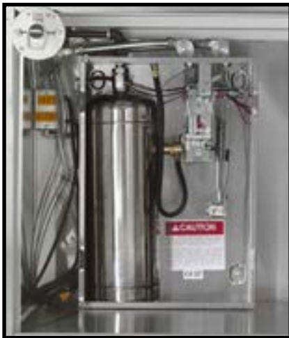
ANSUL canister inside base cabinet
